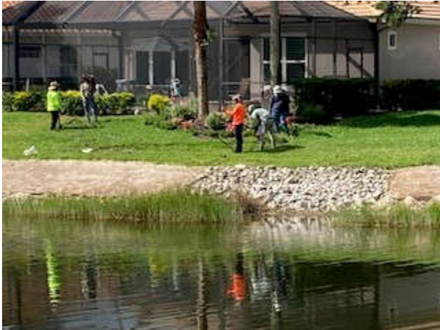
Wednesday, June 14, 2023, Crystal Ct, Lake 38, Irrigation lines/heads install on North shore for Littorals
